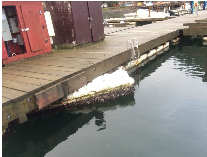
Figure 1. Photo of a burrowed polystyrene dock at Sewell Horseshoe Bay (Photo by Donald Gordon)
